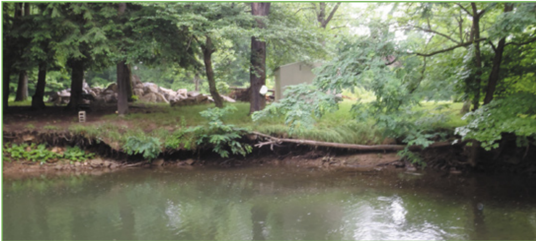
Before: An eroded bank along a section with a nice pool. Tree roots are exposed, the bank is undercut and will collapse into the stream. If nothing is done, the mature trees will eventually be lost, and the stream will become wide and shallow.
